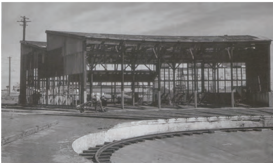
Image 4. The roundhouse during its demolition in December 1970. The five roads under cover are clearly seen with the turntable pit in the foreground. Courtesy Love (1998), p 14.
